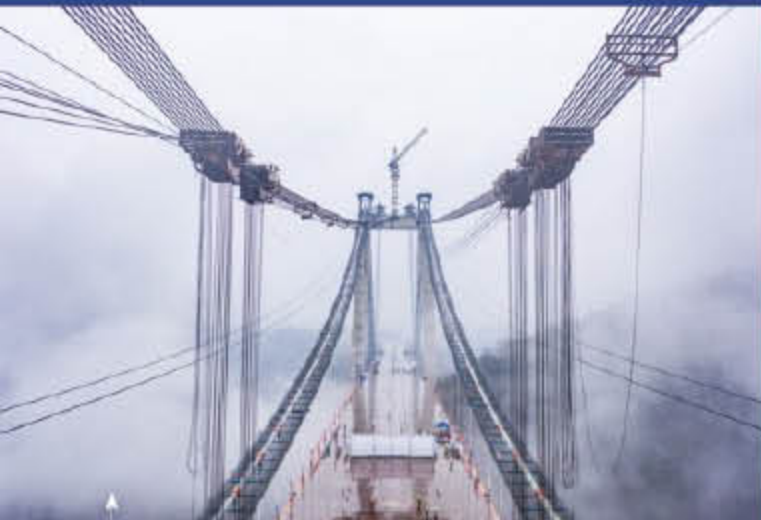
Aerial photo taken on Dec. 29, 2020 shows the Heshandu Wujiang River Bridge under construction in southwest China's Guizhou Province. The bridge, with an overall length of 2,000 meters, is a key project of the Meitan-Shiqian expressway. (Xinhua/Tao Liang)
